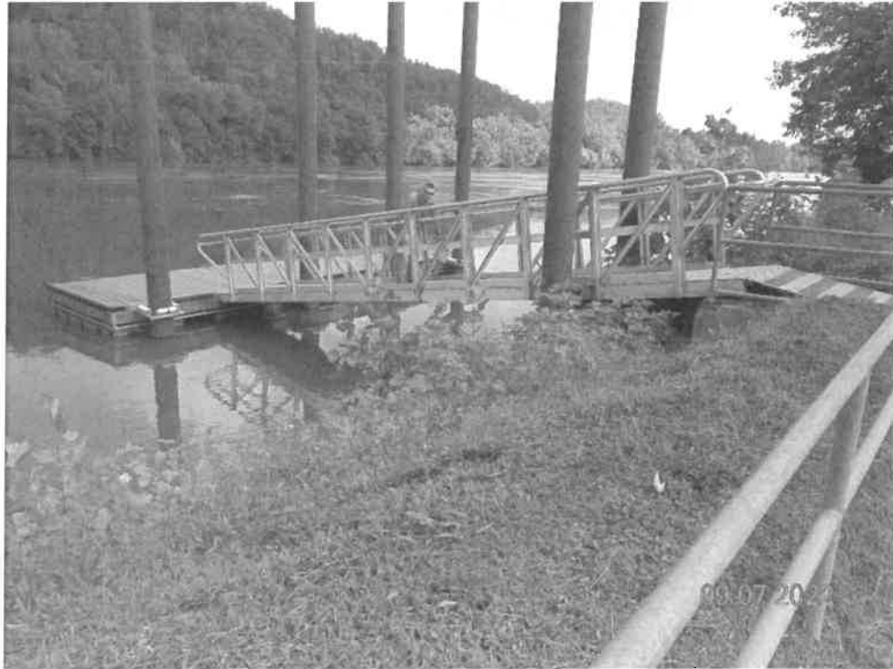
Photo No. 2: Dock and gangway prior to damage in 2022. Note there is a float under the gangway next to the abutment.
