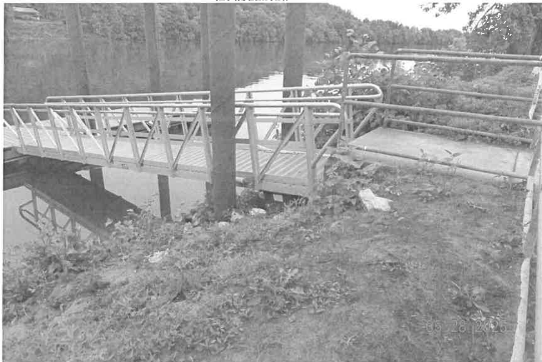
Photo No. 3: The gangway has been shortened to allow the dock to drop back down to normal.
