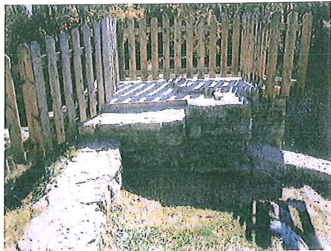
Photo No. 12: The concrete top on the old drain gate well is in good condition. Some of the stone masonry is in need of mortar repair.
