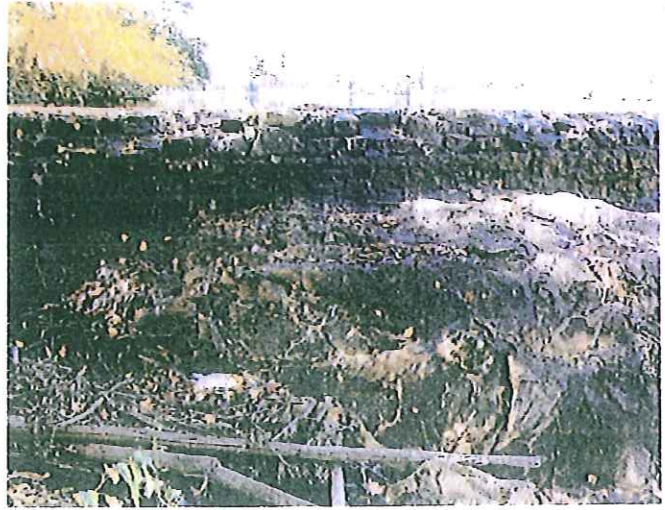
Photo No. 16: Missing spillway stones.
