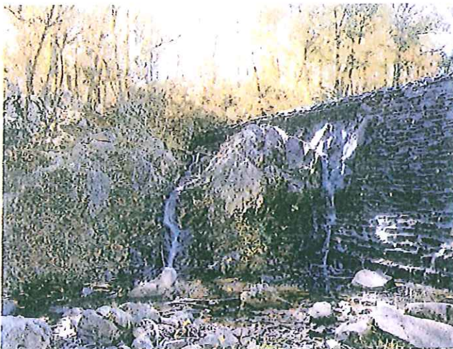
Photo No. 9: Bedrock erosion and old repair along the right end of the principal spillway.
