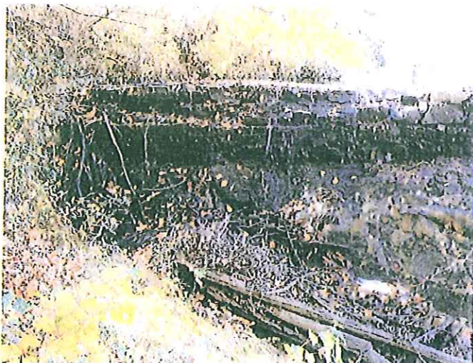
Photo No. 15: Erosion area and missing spillway stones.
