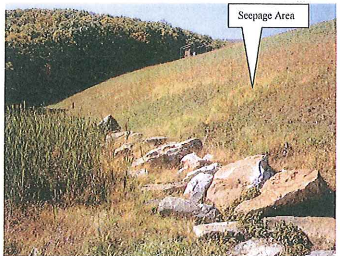
Photo No. 5: Seepage area on the downstream slope near the left groin.
