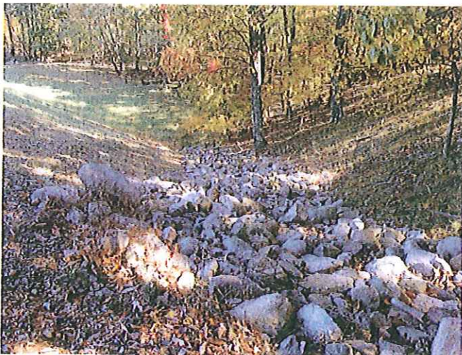
Photo No. 3: New rip rap placed in the right groin where bare soil had been present at the time of our last inspection.
