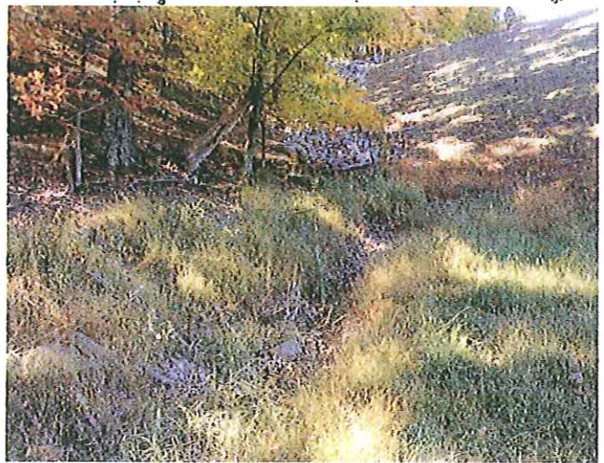
Photo No. 4: Right groin seepage area.
