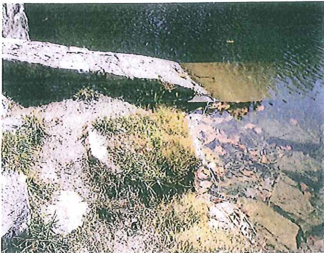
Photo No. 7: Old stump removed and hole filled near the principal spillway guide wall.
