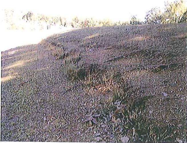
Photo No. 8: Erosion near the right abutment.
