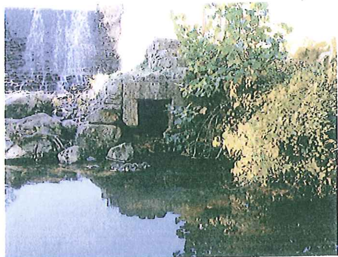
Photo No. 11: Box culvert outlet. Flow was observed on this date even though the gate was closed.
