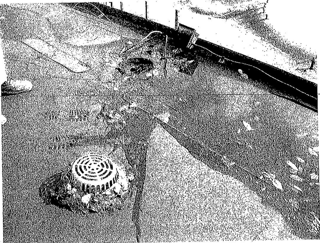
Photo 37. Leaves Blocking Roof Drain
