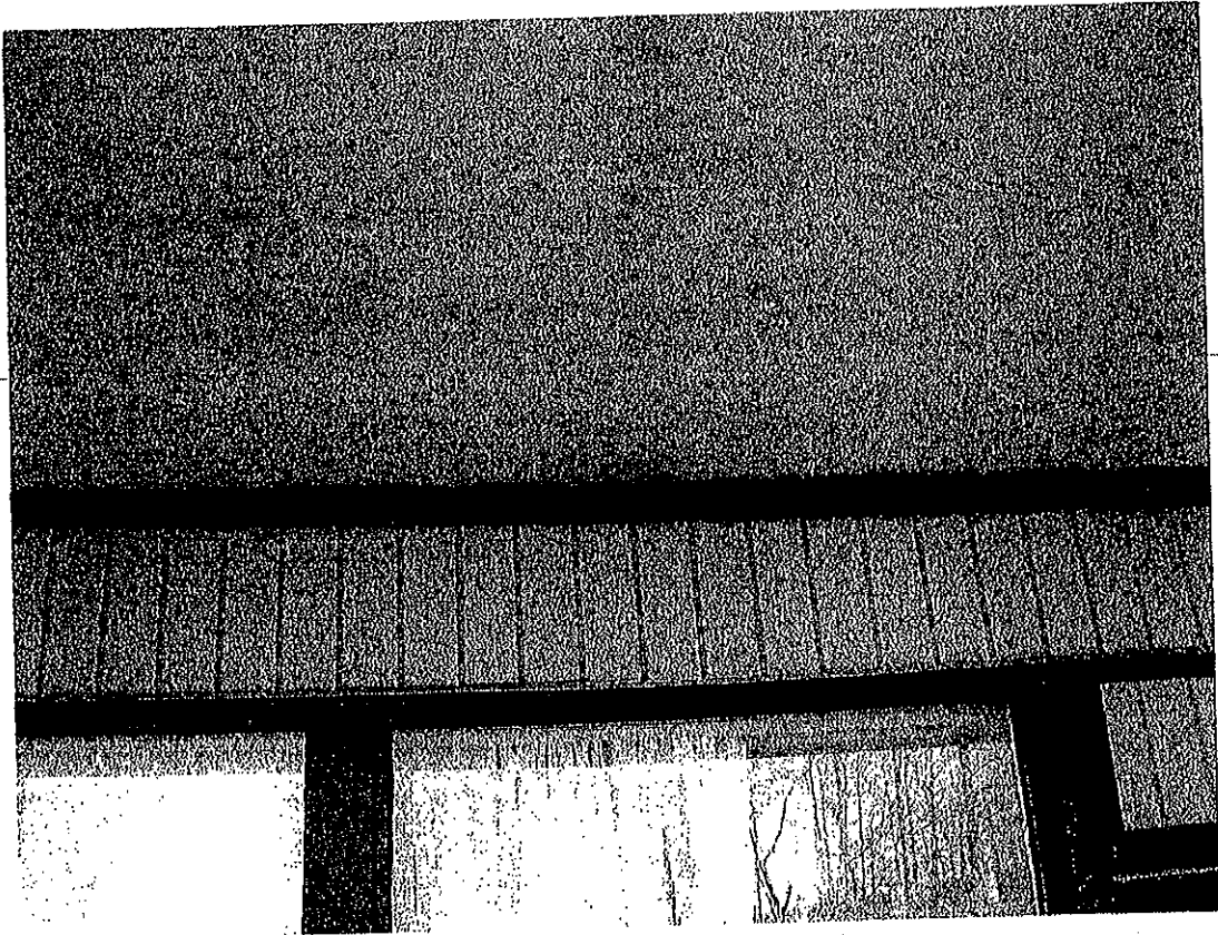
Photo 69. Deflection and Out of Plane Movement of Siding Above Window
