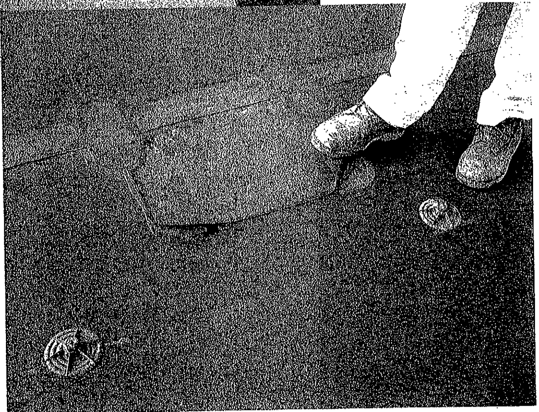
Photo 40. Previous Patches on Roof of Raven Lodge Appear to Be Loose
