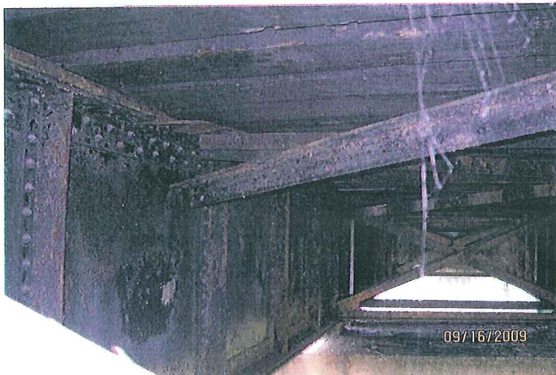
Photo 12 Two top lateral braces are not attached in Span 3.
