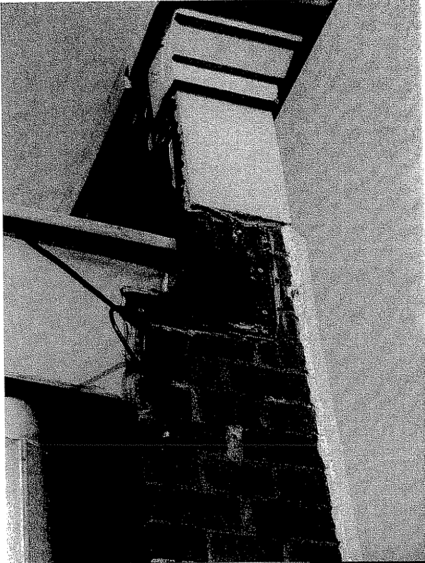
Photo 5. Open Joints Between Upper Roof and Brick Wall that Need to be Closed
