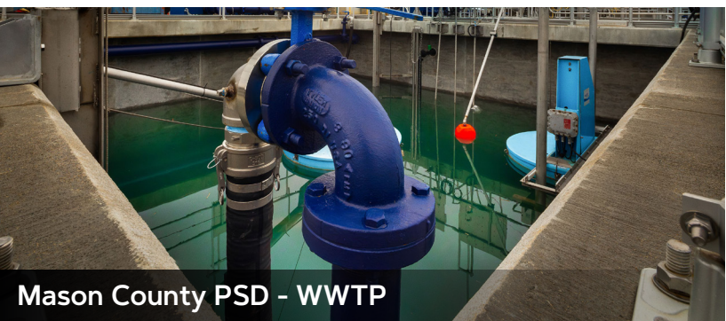
Mason County PSD - WWTP
