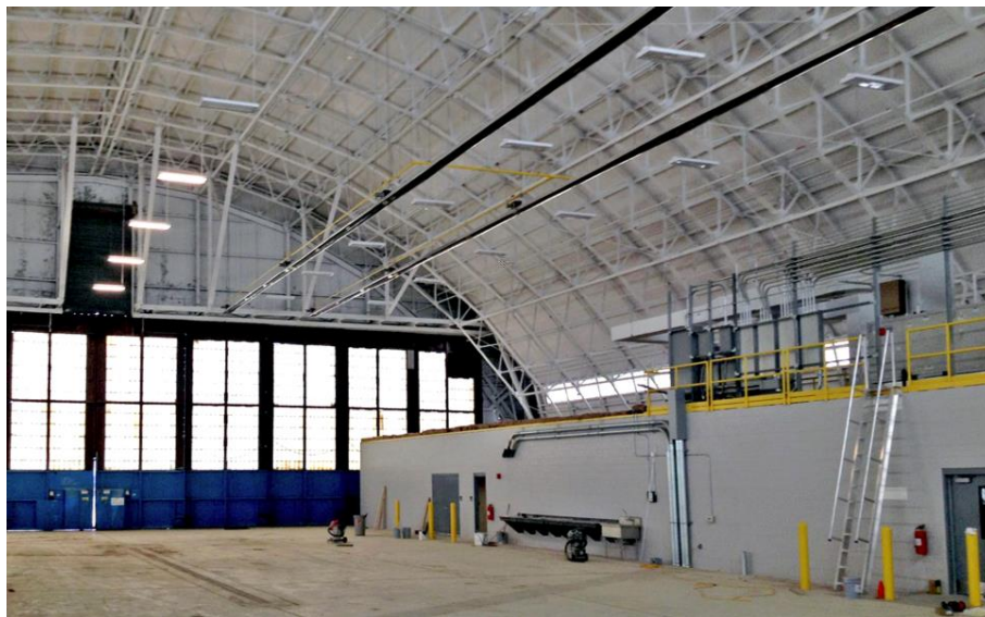
GRW provided design and construction phase services for the WV ANG's 130 th Airlift Wing Building 107 Renovation.
