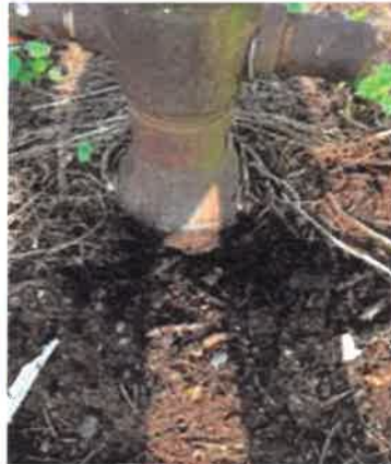
Wellhead Leak Location
