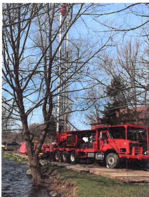
FIGURE 2-4 - PARSONS AND ITS SUB-CONTRACTOR MOBILIZED ON THE ROBINSON WELL, A SITE WITH CHALLENGING ACCESS IMMEDIATELY
