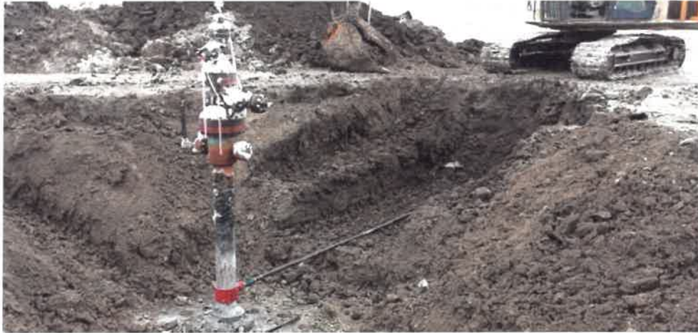
FIGURE 2-2 - VENT SITE CONSTRUCTION. A critical element of these sites is that the methane leak rate is known and measured allowing for comparisons of methane going in versus coming out of the ground
