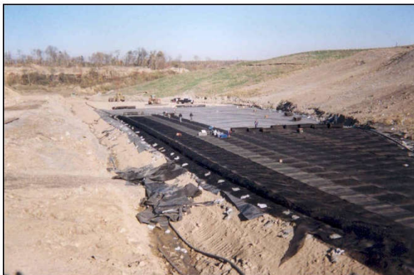
HDPE drainage net was installed as the leak detection layer above the 60-mil HDPE geomembrane.
