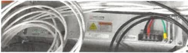
Installed equipment (Batteries)
