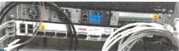
Installed equipment (switch and rectifier)
