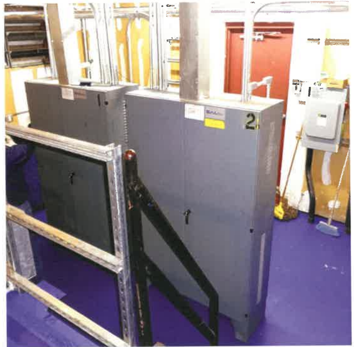
Machine Room After Modernization
