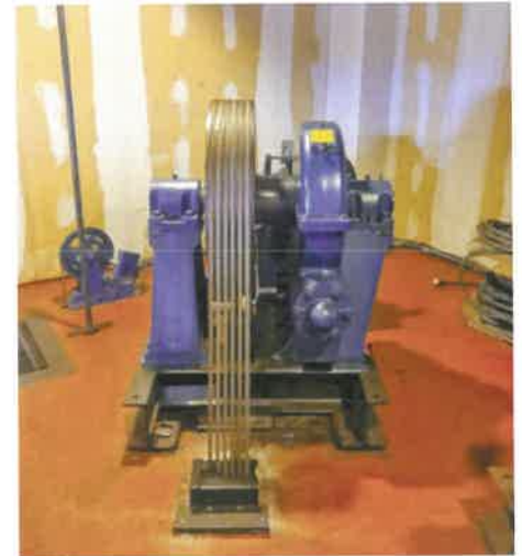
Outdated Equipment Bears Many Risks
