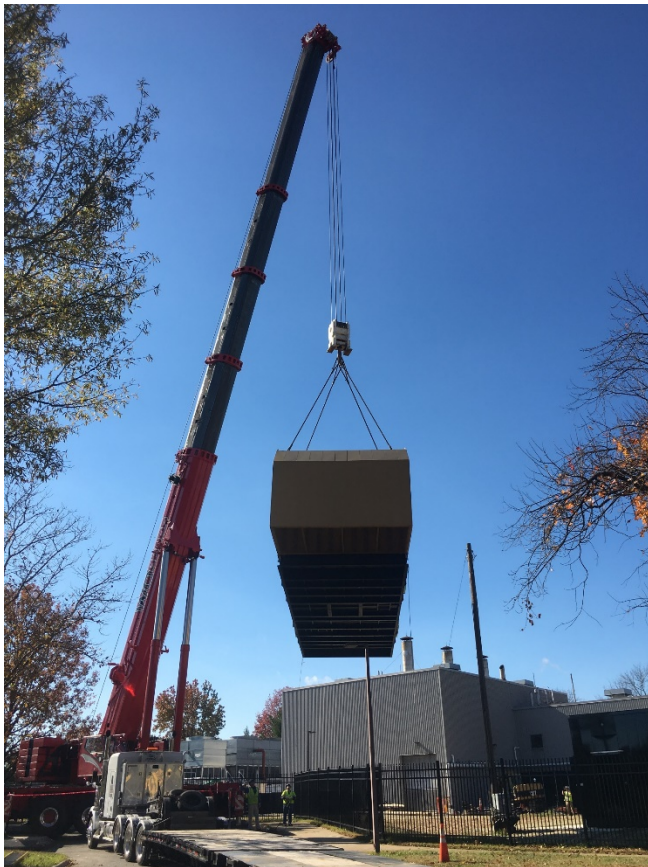
Picture of Setting Fully Assembled Switchgear Building (with switchgear installed) at Richmond VAMC.
