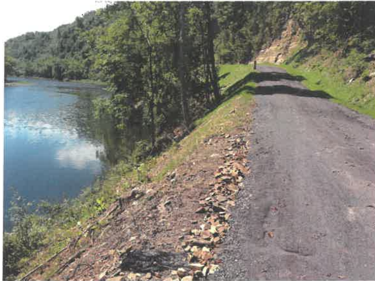
GBRT Slide Stabilized and trail restored.
