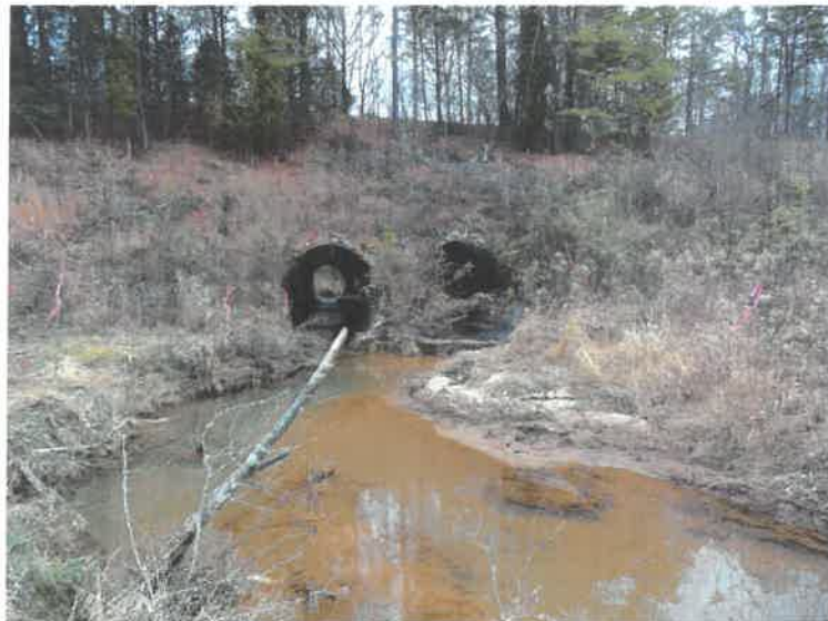
Twin 10 ft. Diameter Culverts & Unstable Embankment
