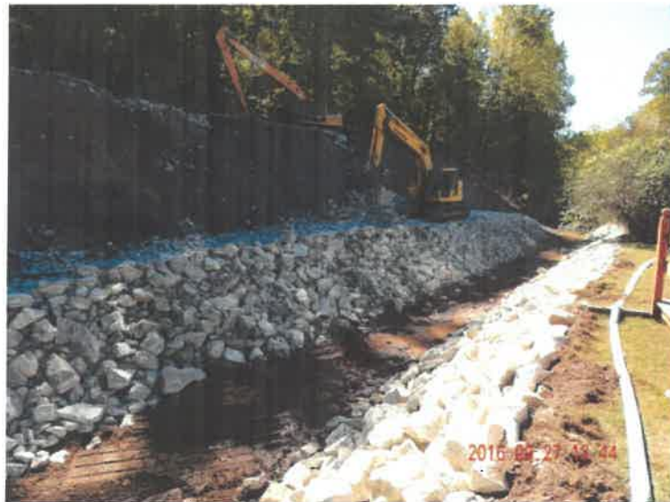
Construction of Rock Toe at NBRT Landslide and Restoration of the Stream Channel
