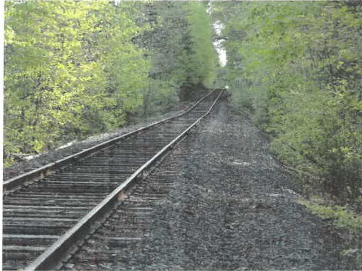
Failed RR Embankment – Duke Energy
