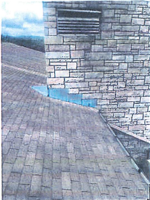
Photo 4: Main building looking back to front showing flashing around chimney.
