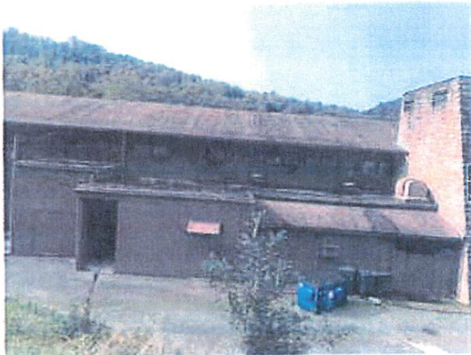
Photo 8: Main building showing flat roof, the various gutter configurations and paper room roof. Note there are gutters on lower portion of paper room roof and along the flat roof above the paper room roof. There are three downspouts on this portion of the roof.
