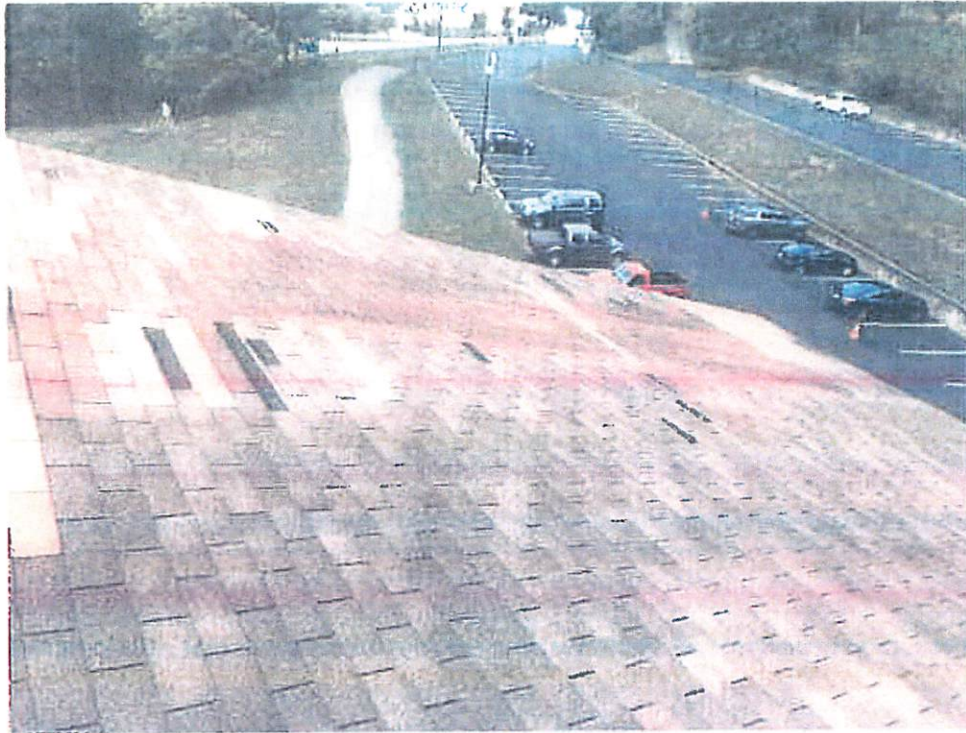
Photo 3: Front right corner of roof showing wind damaged shingle area. This is the only damaged portion of the roof. The sheathing appears to be in good condition.
