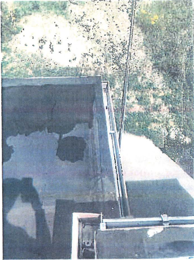
Photo 7: Corner of rubber roof showing various gutter configurations. All guttering will be replaced.
