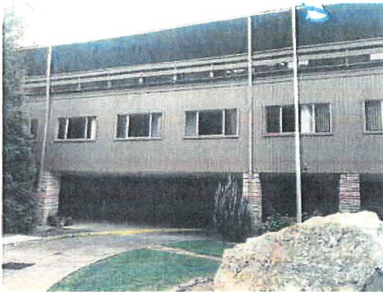
Photo 9: Downspout configuration of front of main building. There are 2 downspouts on this portion of the roof. The second one is hidden behind tree to left.
