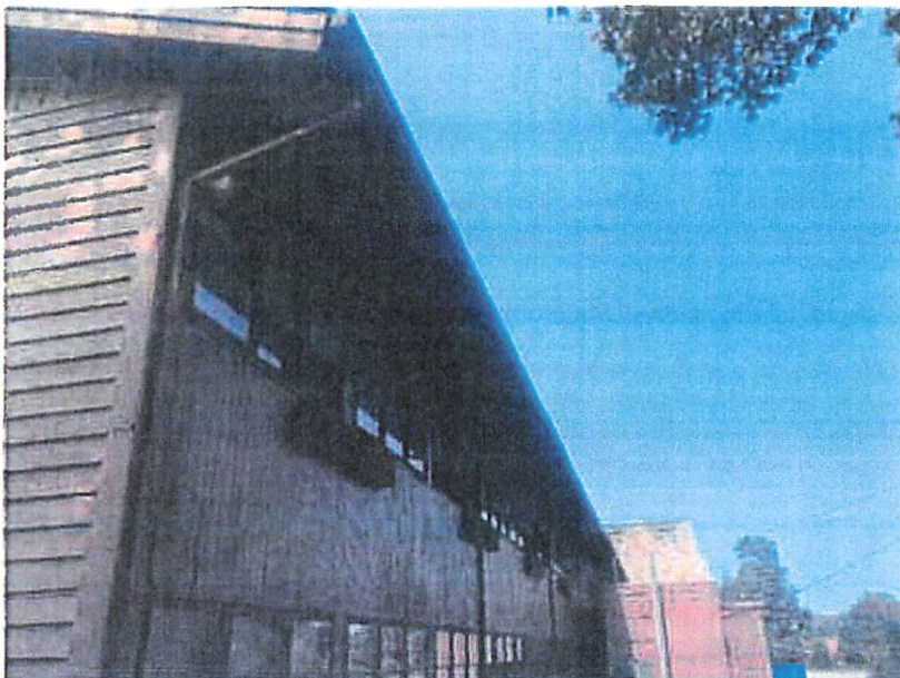
Photo 10: Downspout configuration back portion of front side of building. There are 3 downspouts in this portion of the roof.
