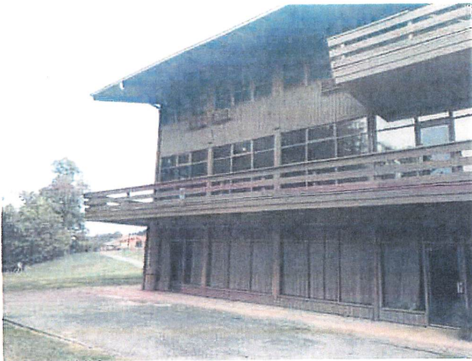
Photo 11: Downspout configuration rear of building (lake side). There are 7 downspouts on rear side.
