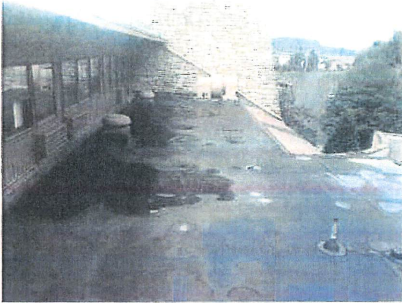
Photo 5: Flat rubber roof showing the small Paper room roof on right. The rubber roof will not be replaced.
