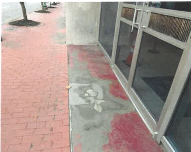
Entry at Lee street is worn and sloping toward the building potentially due to slab jacking.
