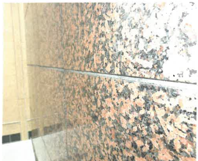
Horizontal joint failure at both upper and lower allow infiltration.
