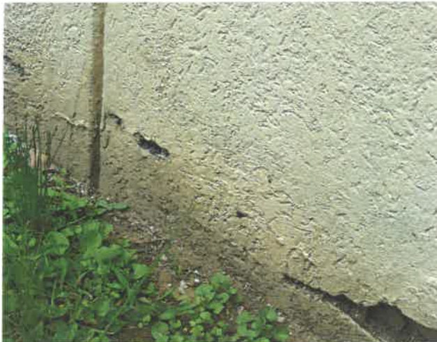
EIFS damage at ground level.
