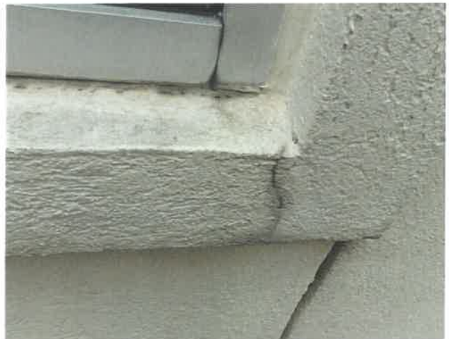
EIFS cracking at windowsills.
