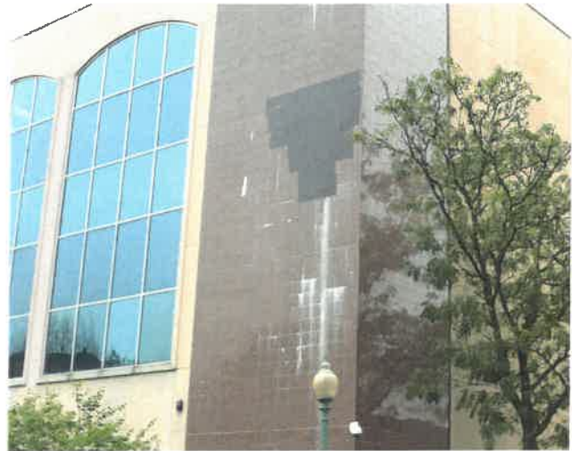
Previously repaired EIF areas at Columns between the banks of windows.
