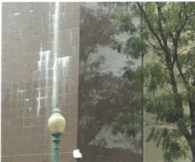
Efflorescence on the tile.
