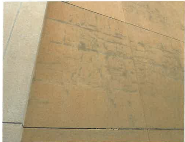
Cracked EIFS on the southern facade.
