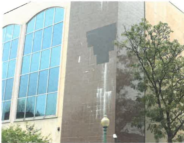
South facade granite tile delaminated and fell from the building.
