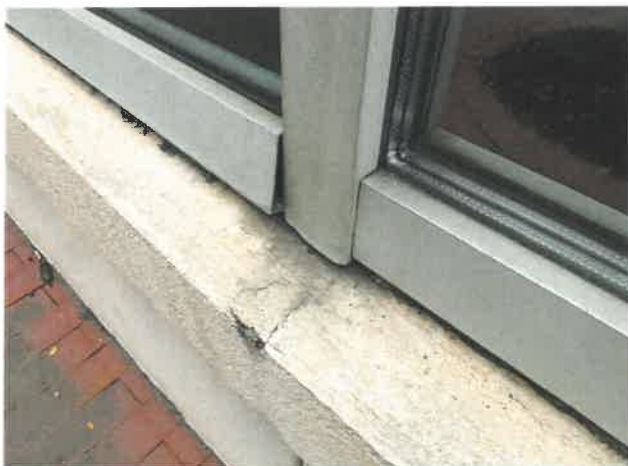
Window trim is detaching in several areas.
