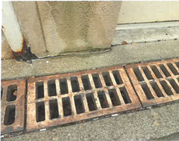
Maintenance of drainage system is required. Steel Doors and frames are corroding.
