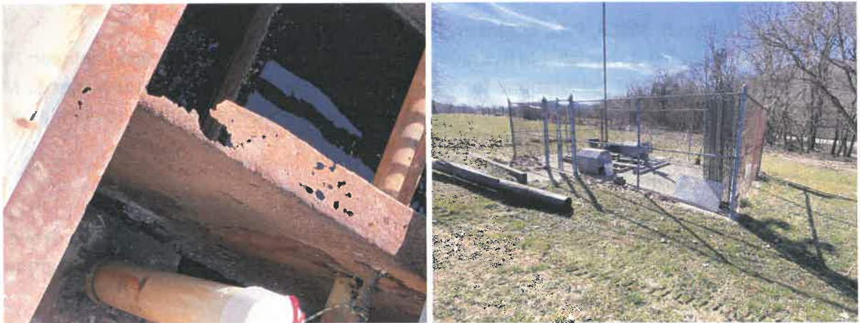
Above left, rust consuming metal parts of the 30-year-old package plant (above right) at the Barboursville School. Photographs by Dunn Engineers Inc.
