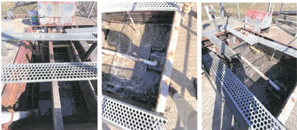
Views of the Barboursville School Package Wastewater Treatment Plant – photos by Dunn Engineers Inc.
