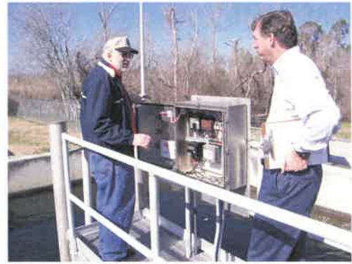
Mr. Hypes (left) as consulting engineer at a wastewater treatment plant in Mississippi after Hurricane Katrina.
