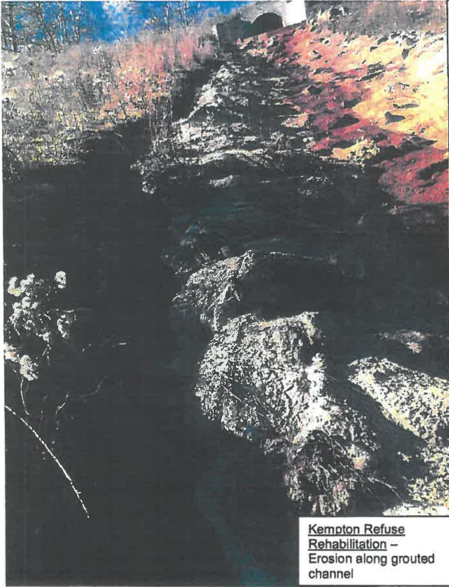
Kempton Refuse Rehabilitation – Grass-lined channel that doesn't convey water
