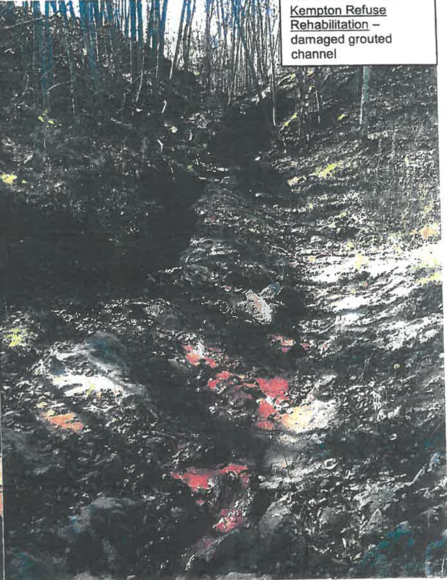
Kempton Refuse Rehabilitation – damaged constructed natural stream
