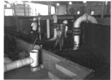
Melvin R. Sampson Fish Production Facility (PRAS 26’ diameter circular tanks for Yakama River Coho Release)
