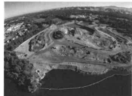
At the Esther Simplot Park D-B Project, McMillen Jacobs moved 250,000 cy of material offsite; total material moved on the project 400,000 cy. Civil works including site grading and storm drains, excavations, extensive dewatering systems, and moving existing utilities.
