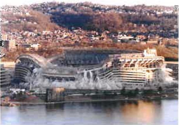
Demolition of Three Rivers Stadium & Engineering Services for Heinz Field Pittsburgh, PA
