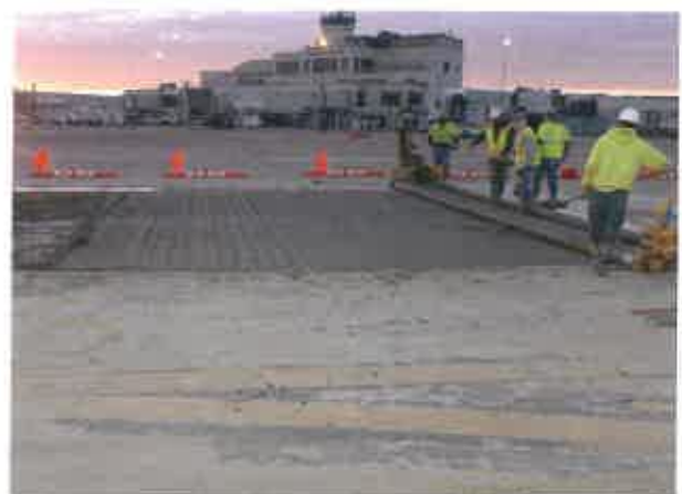
Central West Virginia Regional Airport Authority Taxiway Rehabilitation Yeager Airport, Charleston, WV
