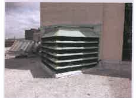
Unique copper louver enclosures to be refurbished
