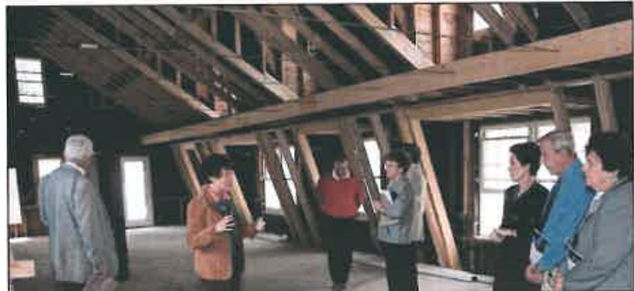
The day lit gallery space is the center piece of this unique adaptive re-use project
