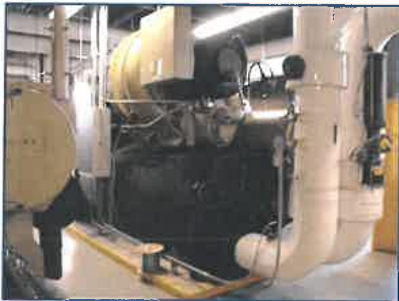
Existing Chiller at Plant
