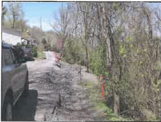
Slide Before Repair
