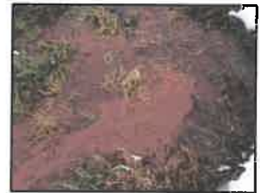
Seepage at a Toe of a Dam
