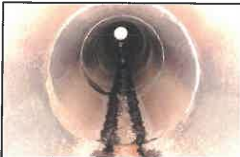
Leakage through Pipe Joints
