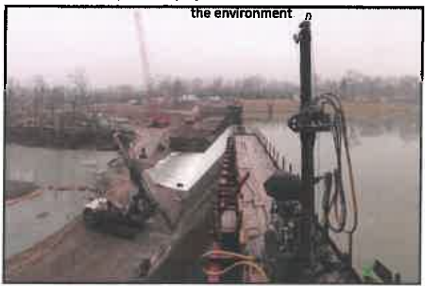
Movable Drilling Platform, Causeway, and Installation of Rock Anchors and Passive Dowels
