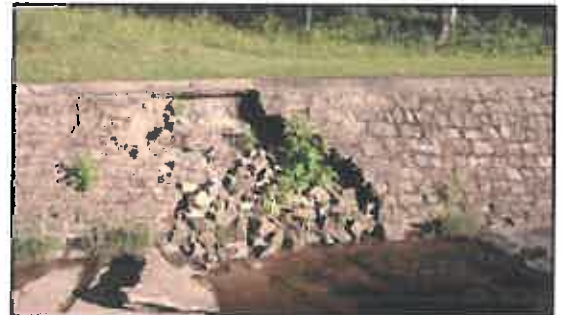
Failure of Stone Training Wall
