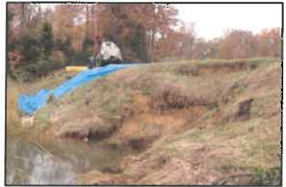
Embankment Slope Stability Issues
