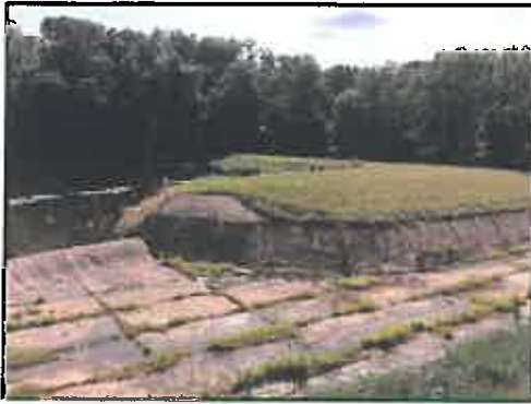
Deteriorated Spillway and Chute
