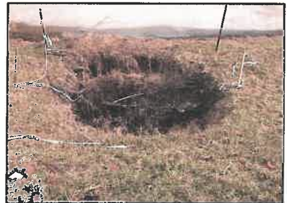
Damaged principal spillway riser and embankment at Dam No. 2
