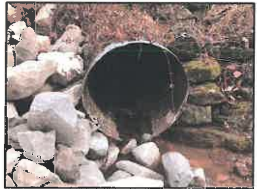
CMP outlet pipe with corrosion along invert at Dam No. 2
