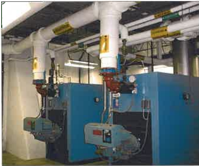
New Boiler Plant
