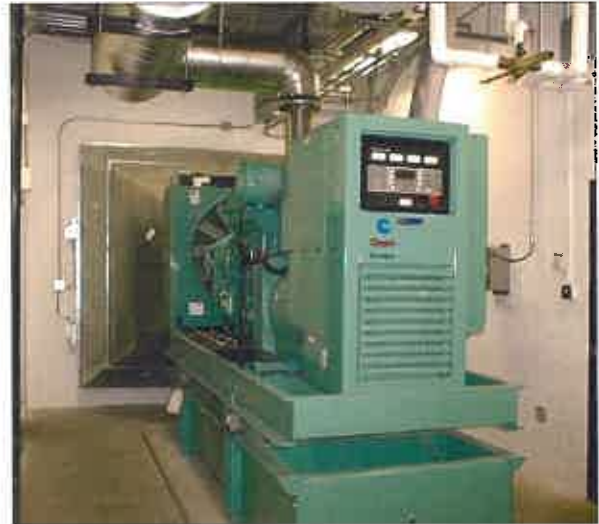
New Emergency Generator
