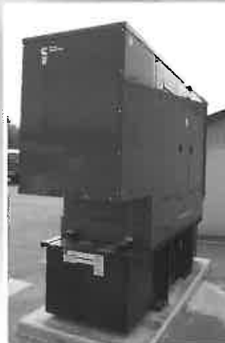
Bus Garage 100 KW Emergency Generator
