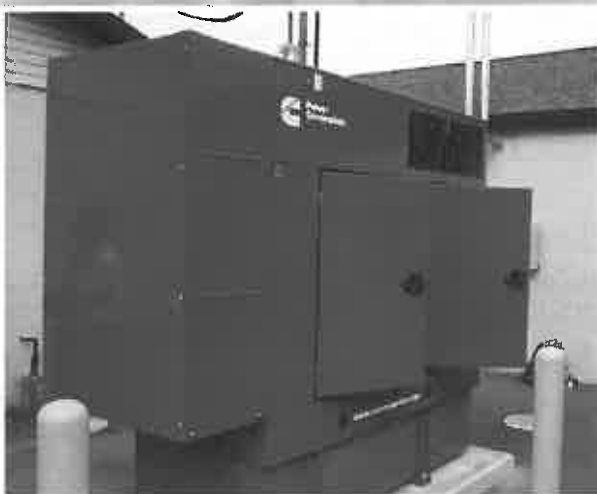
Maintenance Office 60 KW Emergency Generator
