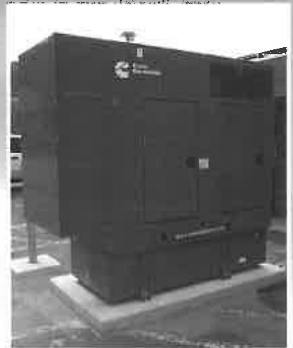
iRaleigh 50 KW Emergency Generator
