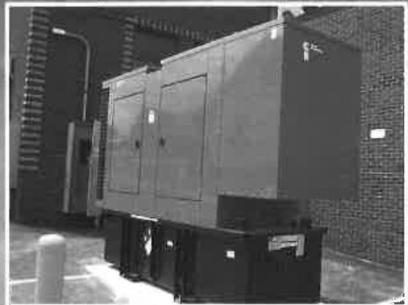
Auxiliary Services 425 KW Emergency Generator
