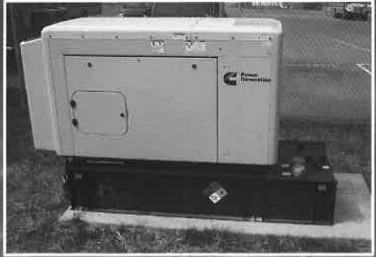
Transportation Office 15 KW Emergency Generator
