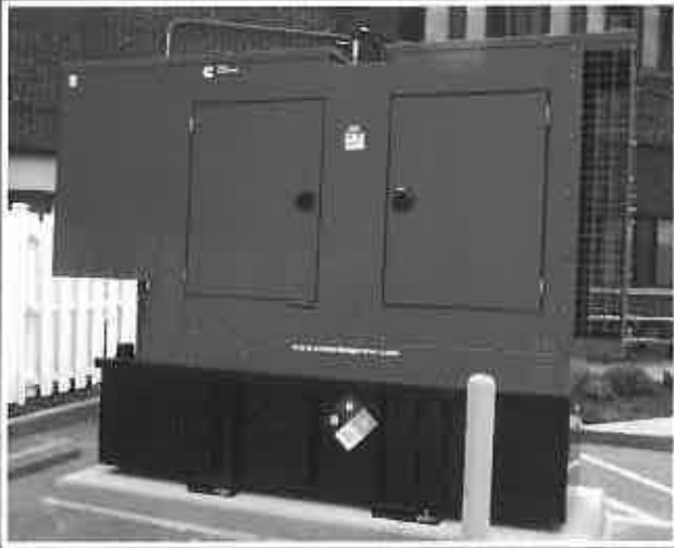
Central Office 100 KW Emergency Generator
