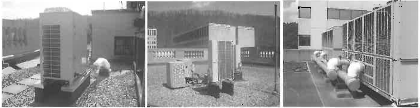
Old Kanawha Valley Bank Building (2003) - New cooling chiller. (2015) - New cooling tower.
