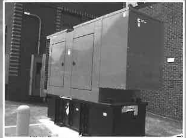
Auxiliary Services 425 KW Emergency Generator
