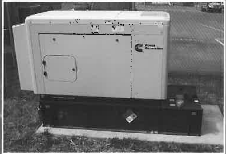
Transportation Office 15 KW Emergency Generator
