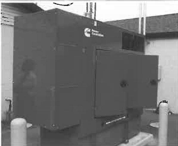
Maintenance Office 60 KW Emergency Generator
