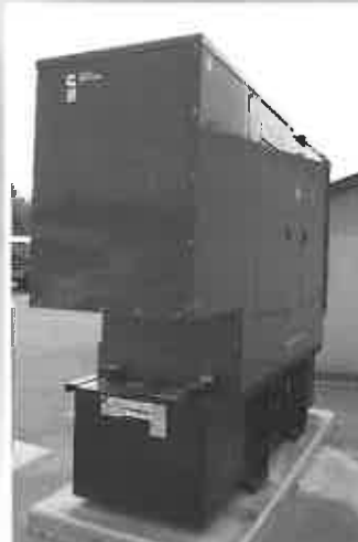
Bus Garage 100 KW Emergency Generator
