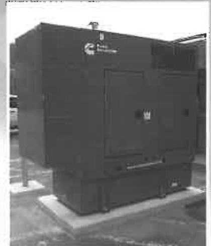
iRaleigh 50 KW Emergency Generator
