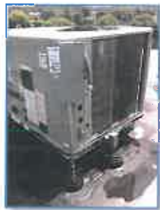
Roof Top HVAC Unit
