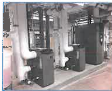
Hot Water Heat Boilers
