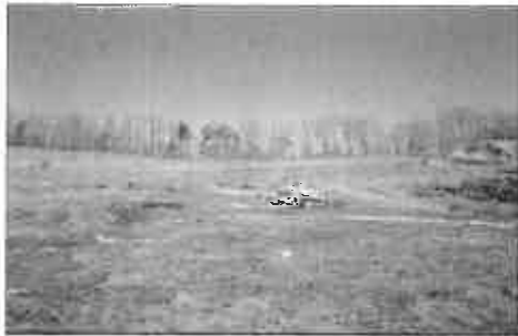
Prior to capping, the landfill area was poorly vegetated and experienced much erosion.
