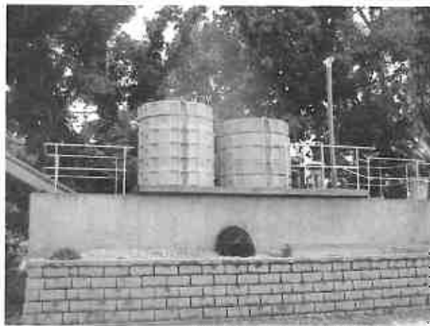
“Headworks” Facility with Scrubber Unit
