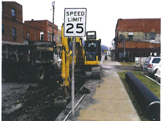
Storm Water Separation on US Route 250
