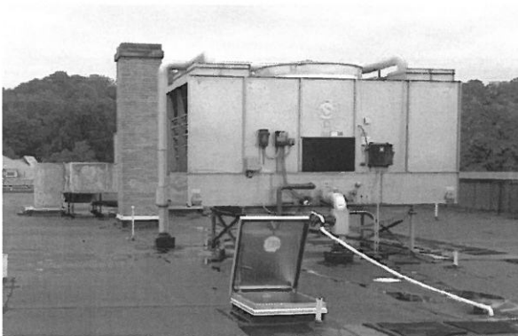
Before Photo - Existing Cooling Tower with Proper Access
