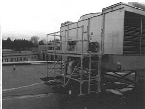
After Photo - New OSAH Approved Ladder and Platform Accessing the Elevated Access Door of the Cooling Unit
