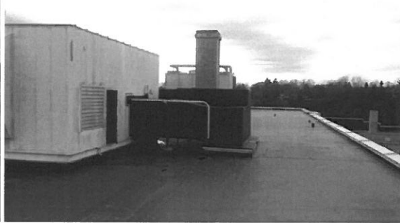
After Photo - Ductwork with Properly Pinned Insulation and Adhered Rubber Membrane
