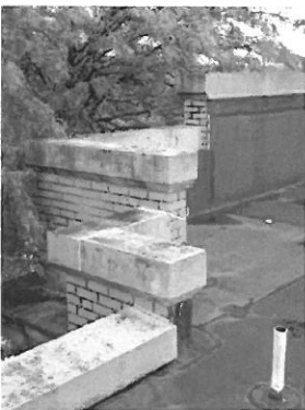
Before Photo - Existing Parapet Wall without Proper Flashing
