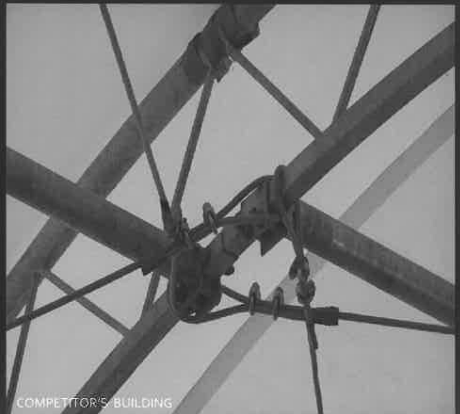
CABLES WRAPPED AROUND SADDLE BRACKETED PURLINS
