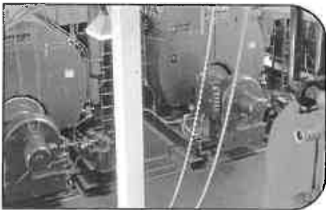
(top) Ruby Memorial Hospital—Morgantown, WV HVAC Exhaust System
