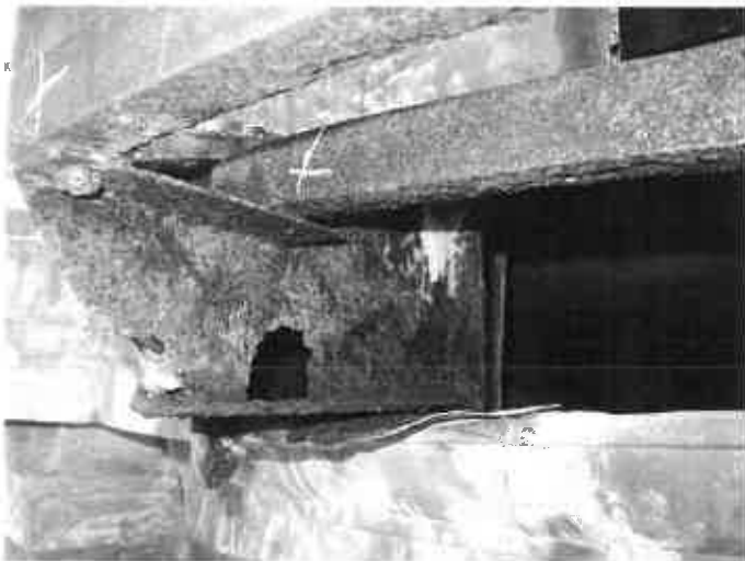
Deterioration of steel supporting sheet metal exhibited such deterioration that portions of the steel have disintegrated.
