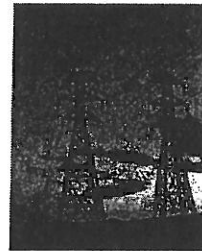
Overhead power lines are un-insulated and can carry tens of thousands of volts, making them extremely dangerous to employees who work in their vicinity.
