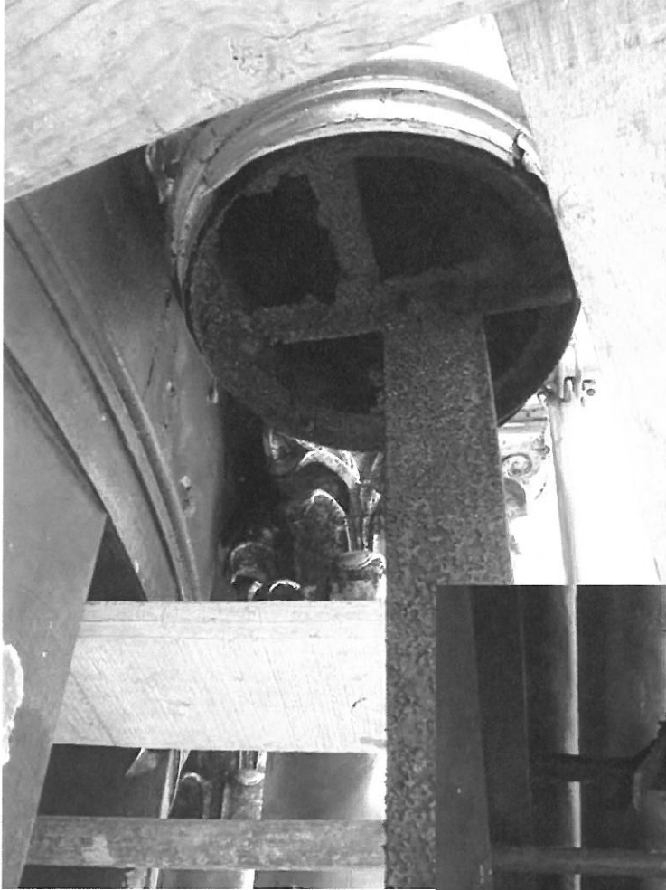
Removal of decorative column wrap indicated that back-up structure was severely deteriorated.
