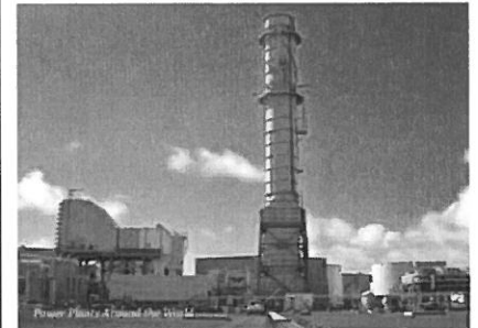
HECO, Campbell Industrial Park
