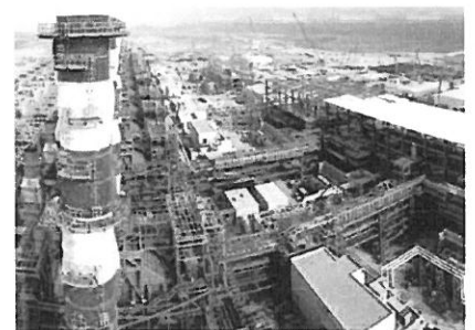
Qurayyah Power Plant
