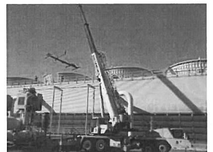
Gila Power Station
