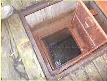
Existing spring box at Spring Run SFH
