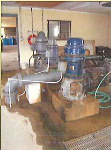
Components of the Reeds Creek Biofiltration & Water Recirculation System
