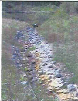
NIXON RUN AMD: Wet Mine Seal outlet pipes and receiving ditch.
