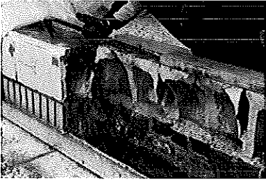
Forensic field investigations revealed significant deterioration of masonry and steel at the terracotta frieze and balustrade.
