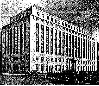
PWWG is leading a comprehensive interior and exterior renovation of historic Building #3 on the West Virginia State Capitol Campus.
