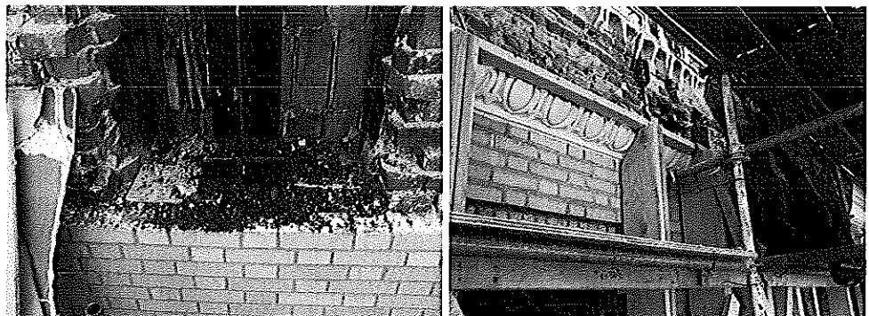
Forensic field investigations revealed significant deterioration of masonry and steel at the terra cotta frieze, balustrade and lintels above the windows.
