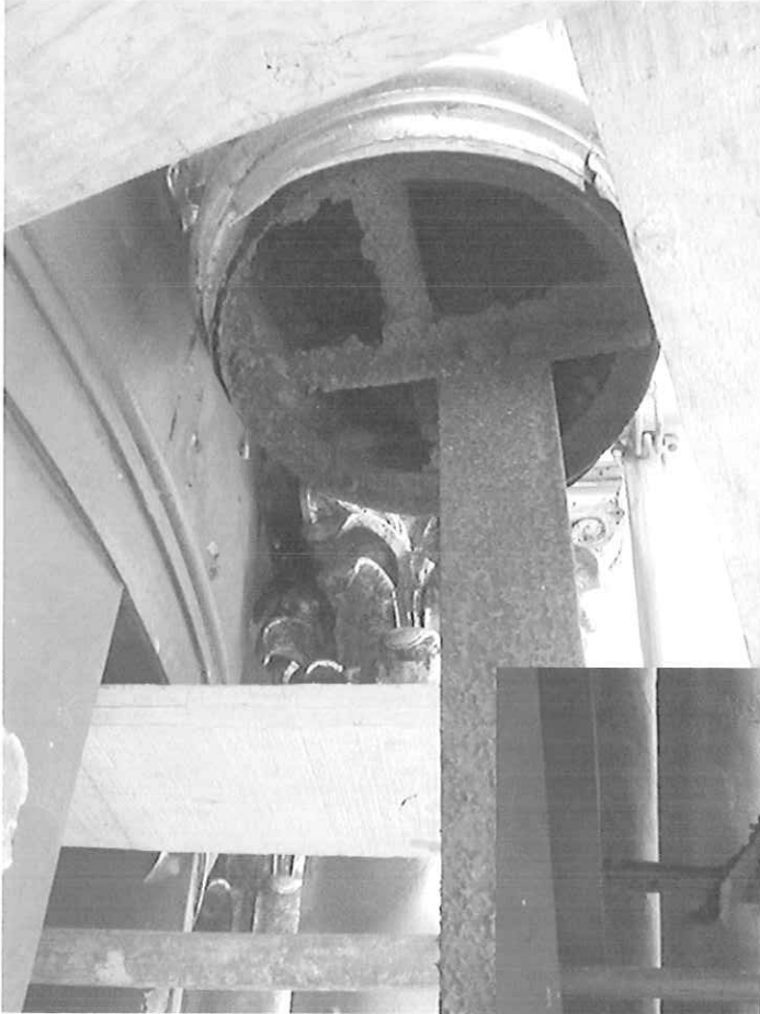
Removal of decorative column wrap indicated that back-up structure was severely deteriorated.
