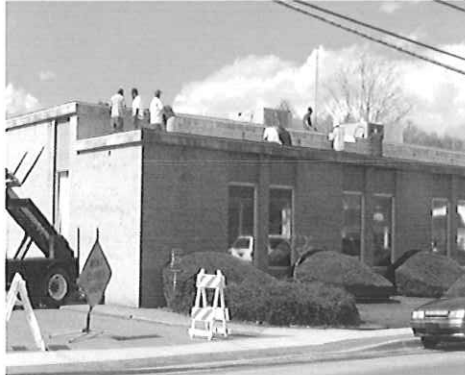
White Sulphur Springs Post Office White Sulphur Springs, WV Reroof Project Completed: 2007
