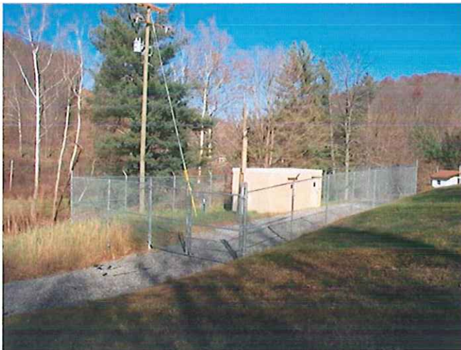
50 GPM Wilsonstown Booster Station
