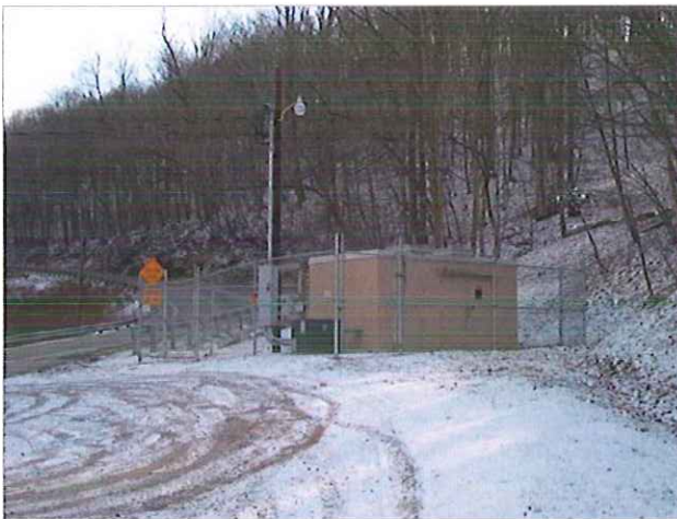
250 GPM Water Booster Station on Route 20
