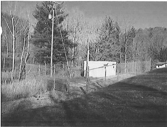
50 GPM Wilsonstown Booster Station
