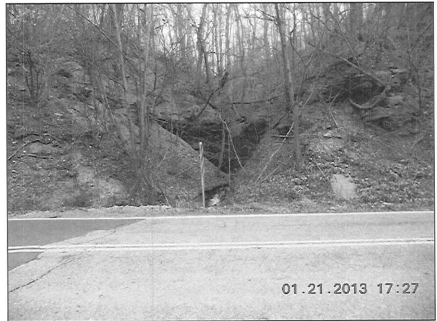
Photo E – Shinns Run – Stream Blockage
