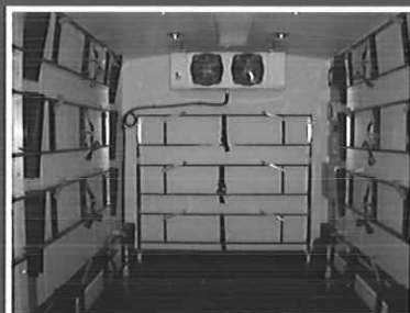
Front Wall / Refrig. Unit
