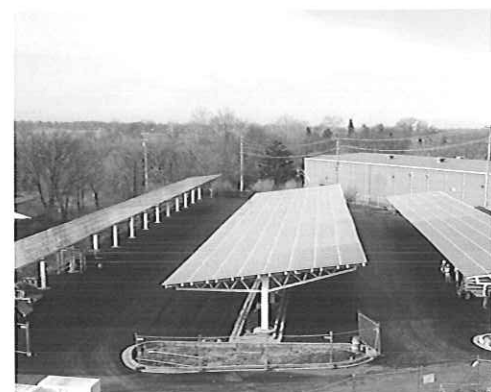
Solar array / parking lot shading
