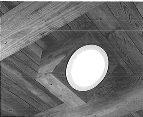
Solatube daylighting system
